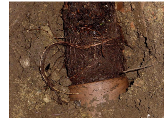
Drain full of roots
