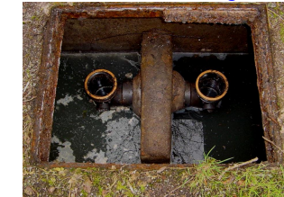
Good condition dip-pipes
