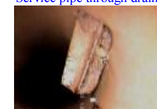
Fence post through drain
