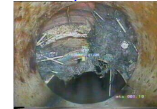
Drain full of roots
