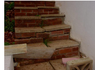
Damaged by leaking drain
