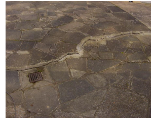
Cracked by leaking drain
