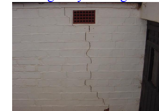
Cracked due to leaking drain
